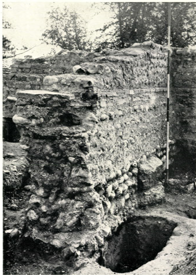
Fig. 2. Site III. E. wall of room 6, 2nd house. A. ground level when wall was built; B. double lacing course of tiles, p. 16
